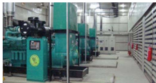
Project: Sommerset Centre TD Hai Phong Package: Backbone Power System Client: Ascott Group Value: 15 billion VND Time: 2015
